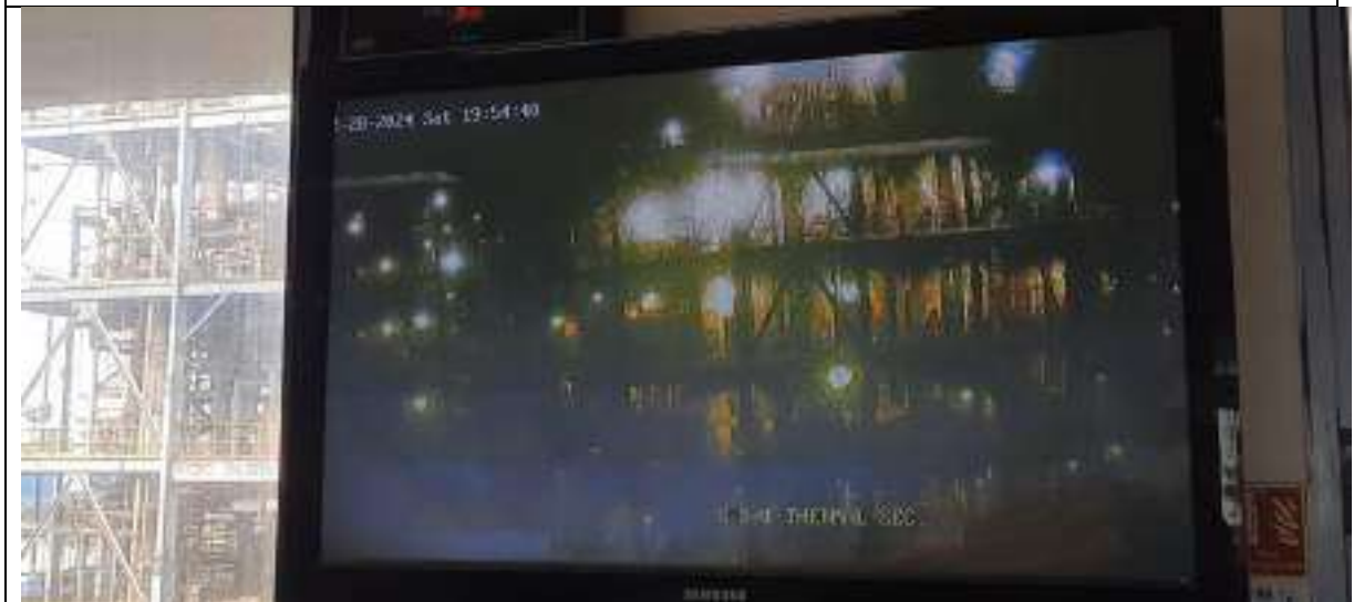
Photographs of CCTV camera located on Control Room of CMS plants in front of CMS-1 plant.
