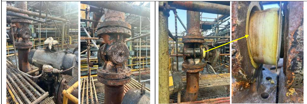
Photographs of damaged valve (DISH visit after incident)
