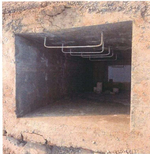
Trench and Drain for Leachate
