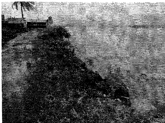
a. Eroding road leading to the entry gate of the proposed port
