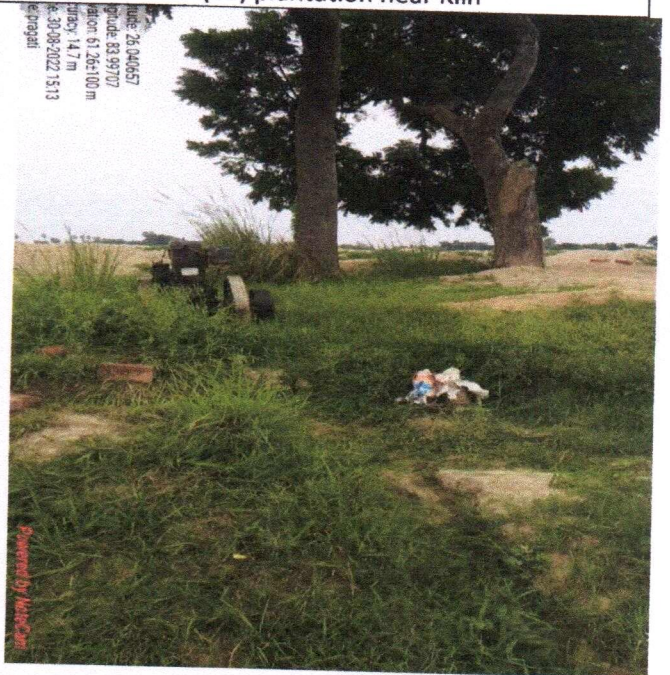
Pic. (04) Diesel Engine for Ground water extraction
