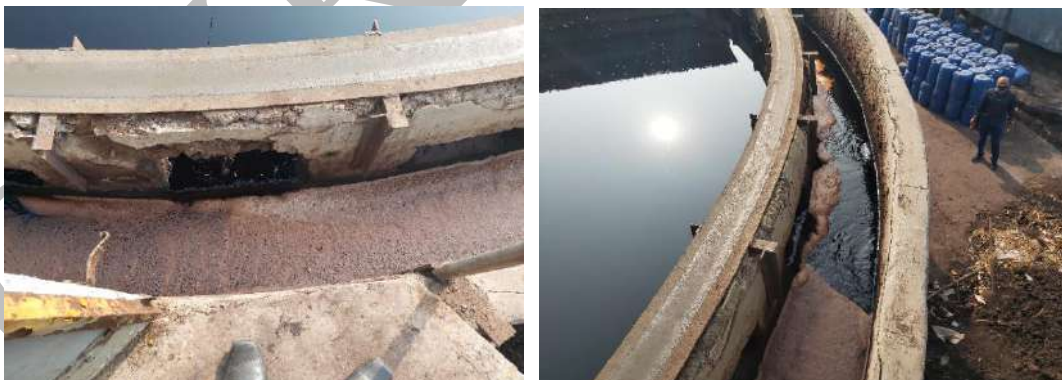
Figure 7.6: Primary clarifier without weir and damage structure
