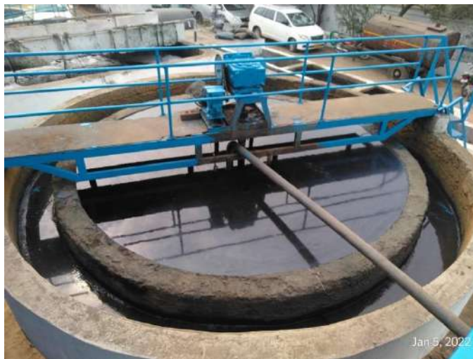
Figure 6.6: Primary clarifier without effluent weirs at CETP Narol Dye Stuff
