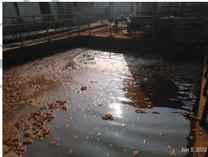
Figure 5.4: Floating and accumulation of solids in equalisation tank
