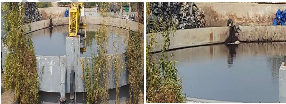
Figure 7.13: No weir installed in secondary clarifier –
