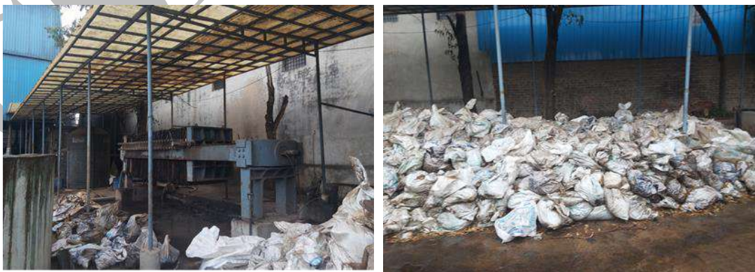
Figure 9.8: Picture showing plate & press filter and dewatered sludge stored at CETP premises
