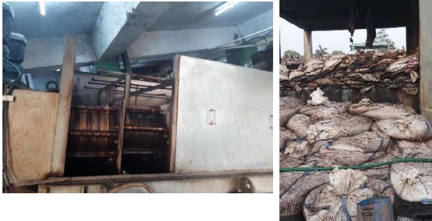
Figure 7.14: Volute automatic screw & chemical and biological sludge stored in CETP premises
