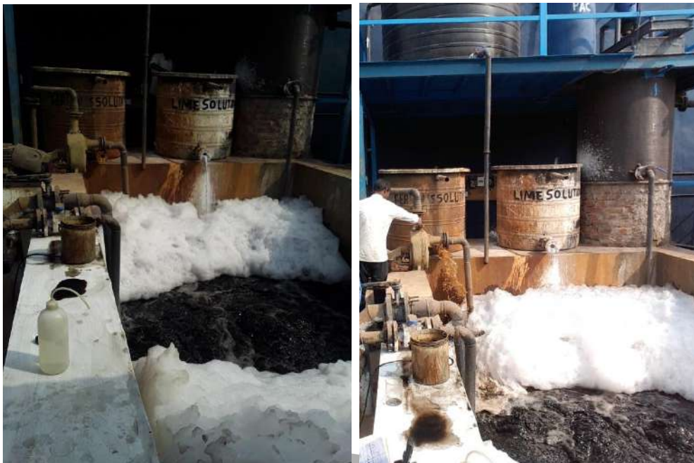
Figure 6.4: Lime and ferrous sulphate dosing in equalization tank at CETP Narol Dye Stuff
