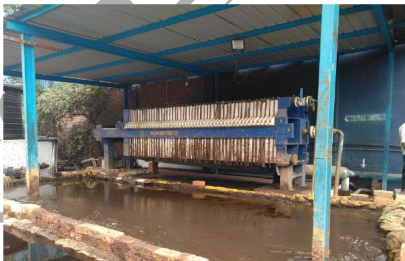
Figure 6.5: Filter press for dewatering of physico-chemically treated effluent at CETP Narol Dye Stuff
