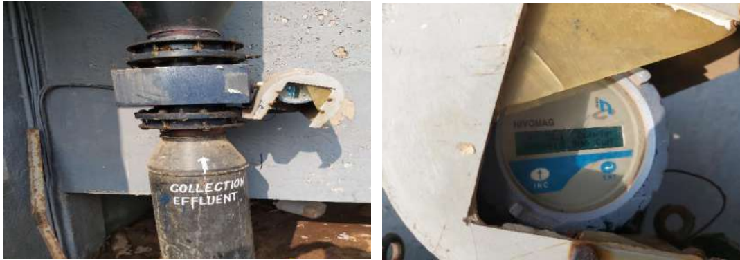
Figure 7.5: Flow meter installed between collection tank – I and flash mixer unit
