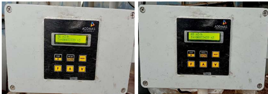
Figure 9.5: Flow meter installed before physicochemical treatment
