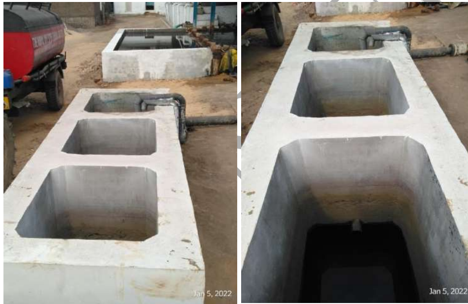
Figure 6.3: Oil and Grease trap without baffles or Upward piping discharge at CETP Narol Dye Stuff
