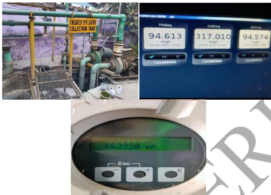
Figure 8.7: Online monitoring system and flow meter
