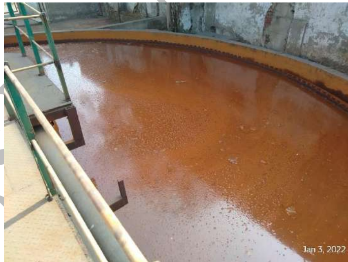
Figure 5.6: Floating solids in secondary clarifier due to irregular de-sludging and recycling
