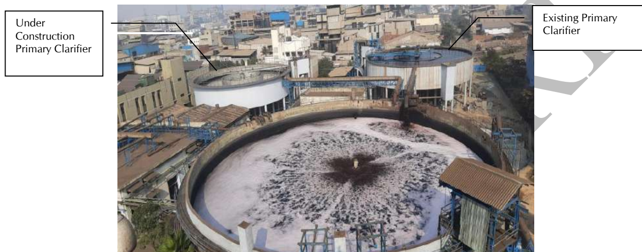
Figure 4.4: Single Floating aerator in Equalisation Tank and under Construction Primary clarifier
