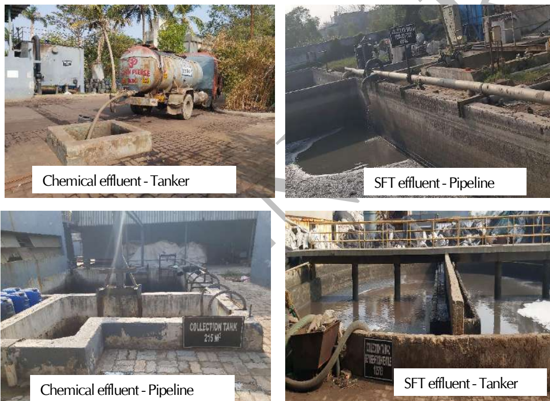
Figure 7.4: Effluent received in CETP trough tankers and conveyance system
