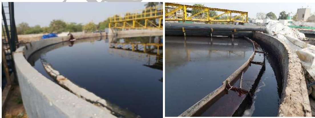
Figure 7.17: No weirs are provided in secondary clarifier
