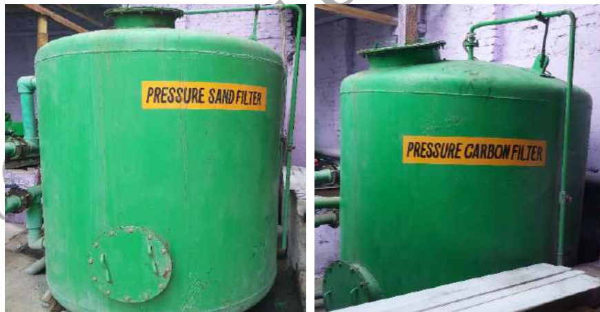
Figure 8.6: Pressure sand filter and pressure carbon filter
