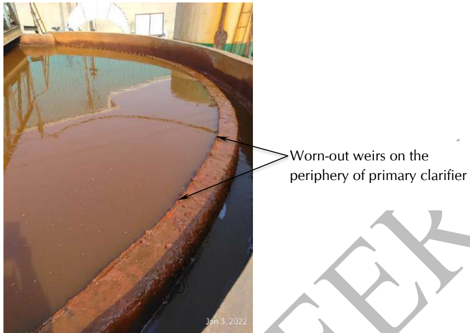
Figure 5.5: Picture showing worn-out weirs in Primary Clarifier
