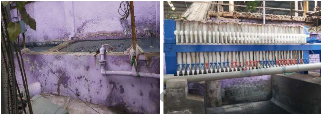
Figure 8.5: Sludge drying beds and filter press
