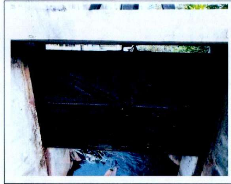
HALISAHAR DRAIN LOCKGATE
