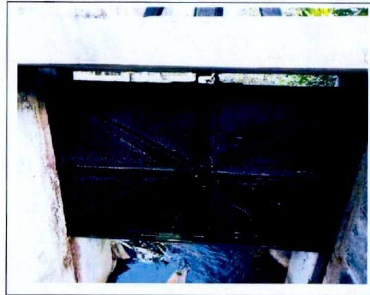
HALISAHAR DRAIN LOCKGATE
