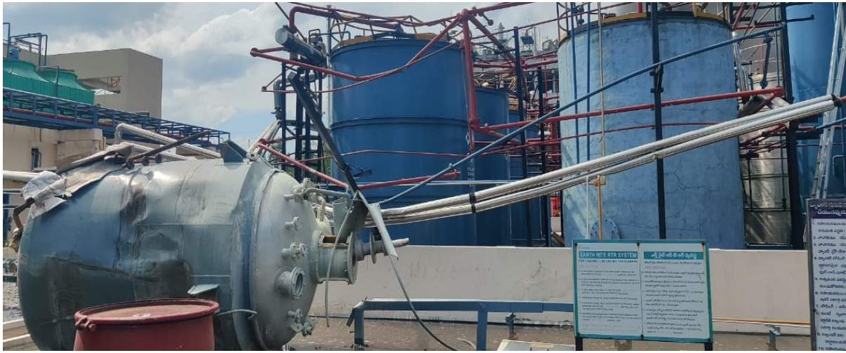
Exploded Distillation Reactor of Sahithi in adjacent Laurus unit-6.
