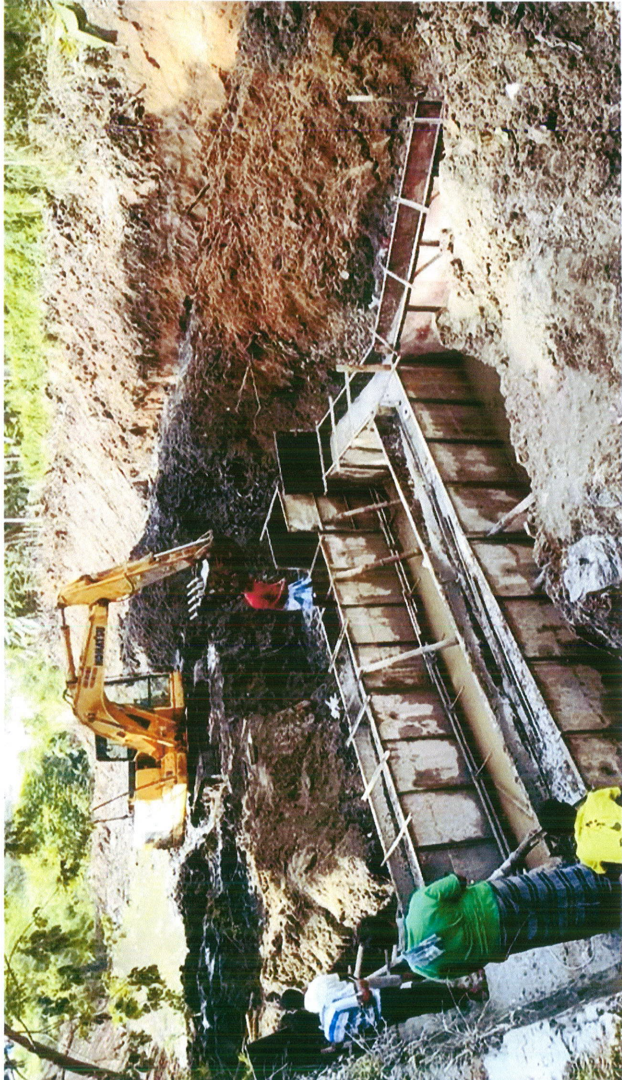
COIMBATORE DISTRICT - NO.04. VEERAPANDI TOWN PANCHAYAT Bio-remediation Techniques Phytoremediation, Constructed with Wellands in Ward No.2 Burial Ground Near pallam Estimate cost Rs.4.20 Lakhs
