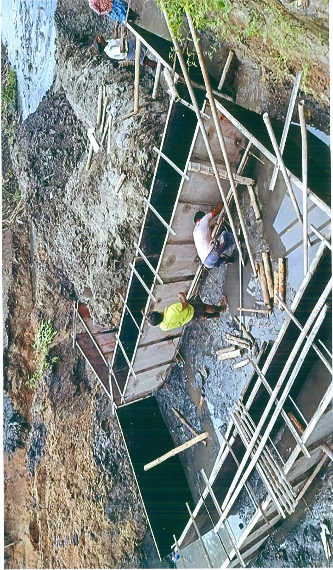
COIMBATORE DISTRICT - NO.04.VEERAPANDI TOWN PANCHAYAT Bio-remediation Techniques Phytoremediation, Constructed with Wellands in Ward No.2 Burial Ground Near pallam Estimate cost Rs.4.20 Lakhs
