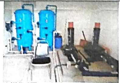
60 KLD STP provided within the apartment premises towards North-West corner of the apartment.
