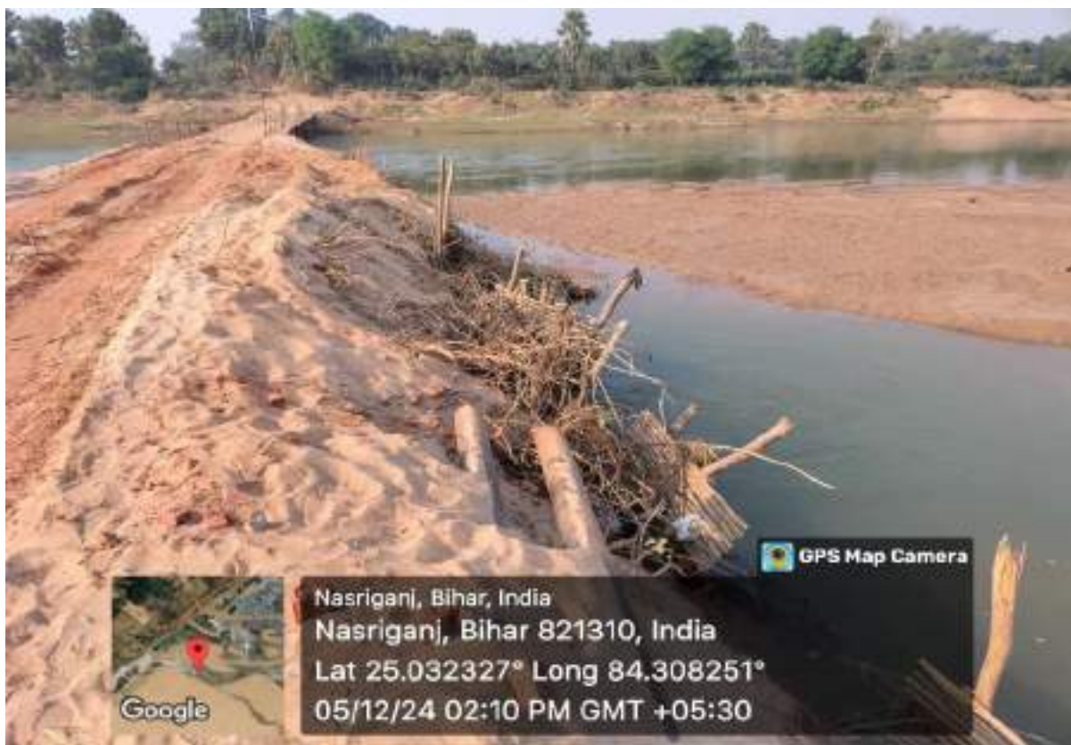
Pic 8: Restricted flow at sand structure and unrestricted flow under iron bridge at Block No. 5
