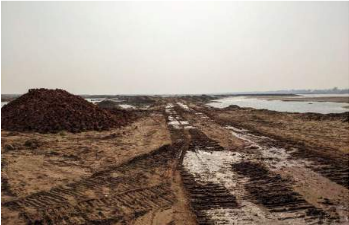
Pic 5: Excavator tread marks at Sand Block No. 5
