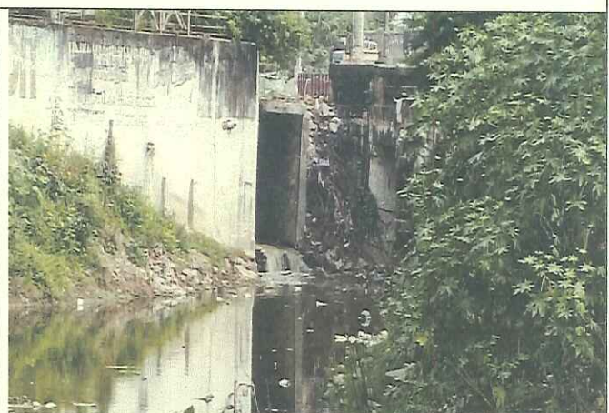
Discharge of sewage from Kelkattalai, Moovarasanpet and Madipakkam Area
