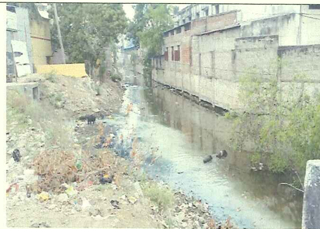
Discharge of sewage from Nanmangalam Area
