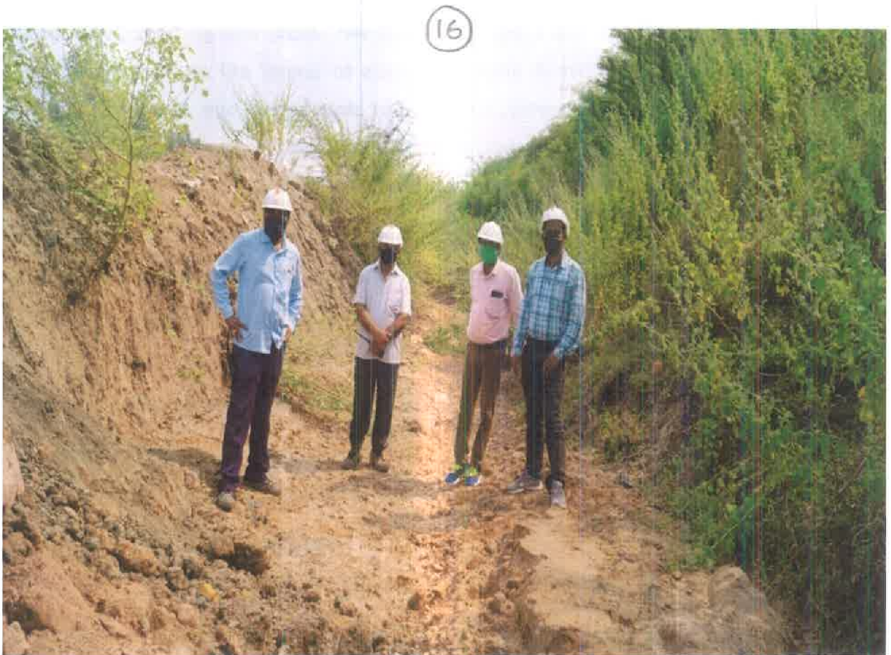
Garland drain along D-3 Dump
