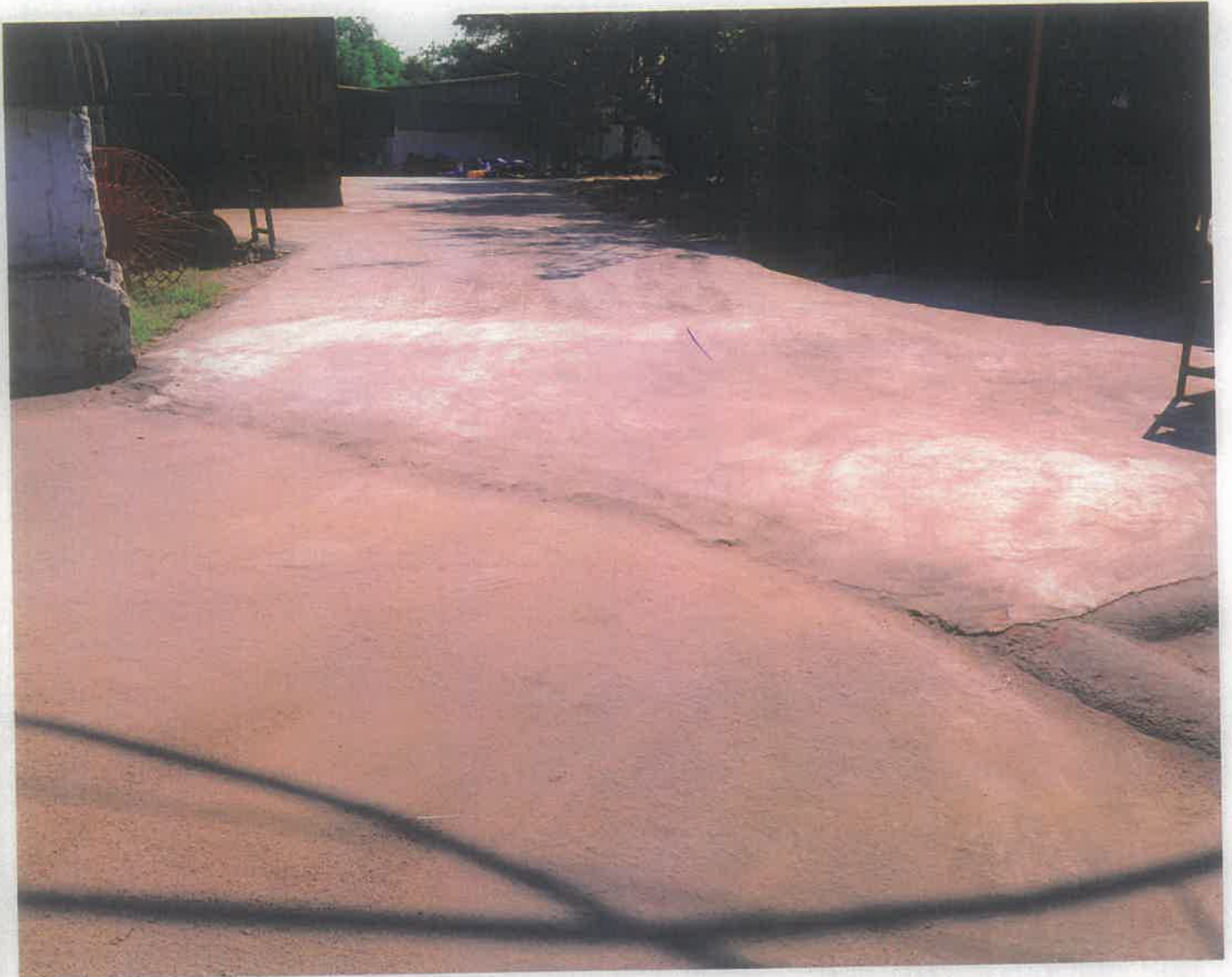
Paved Concrete Road For The Entire Vehicle Movement Area To Control The Fugitive Emission
