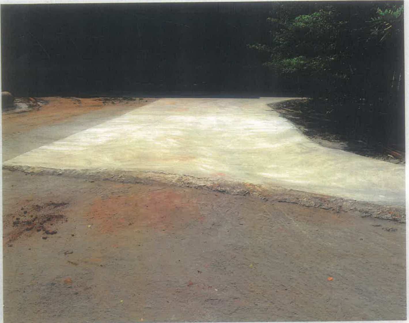
Paved Concrete Road For The Entire Vehicle Movement Area To Control The Fugitive Emission
