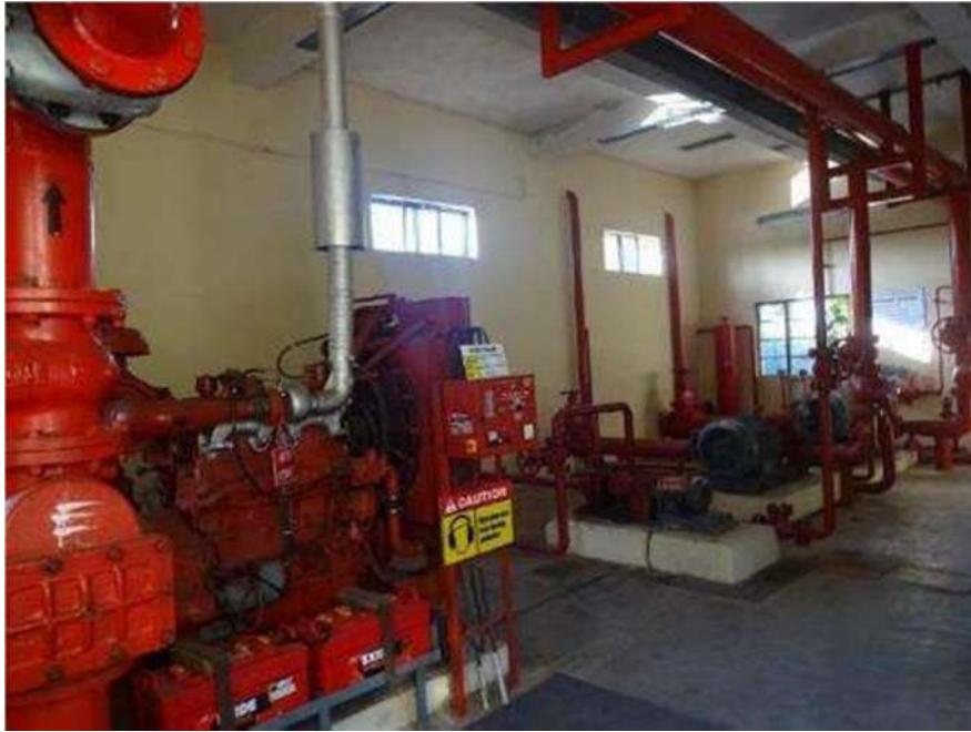
Full automatic Fire Hydrant station – Capacity
