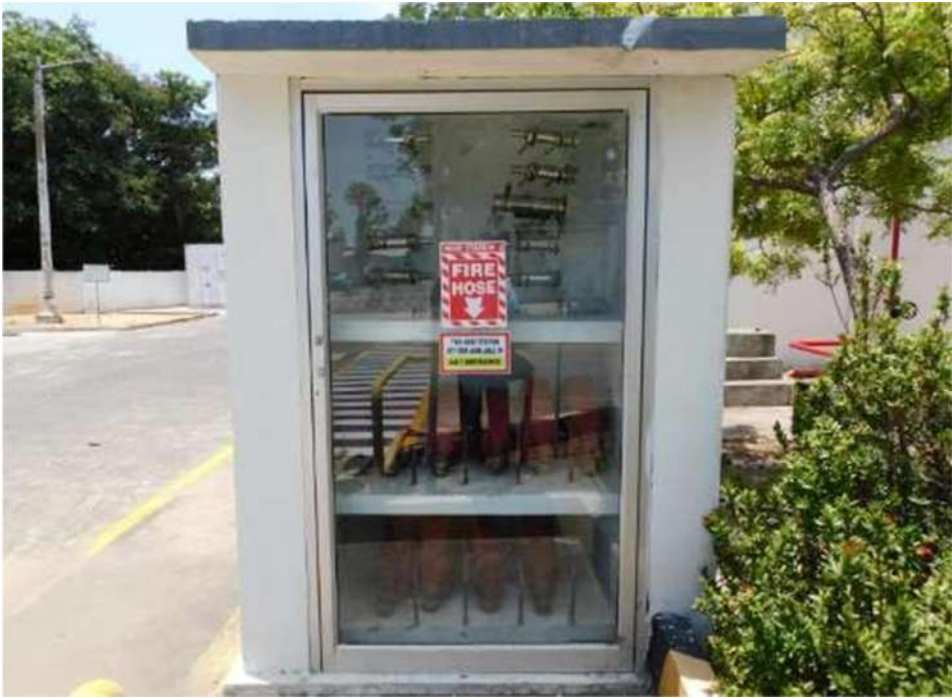
Centralized Hose station & Nozzles- 6 Locations
