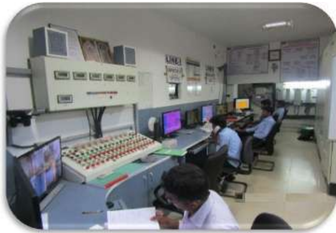
DCS- Automatic Operation station
