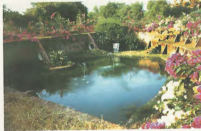
Waste water treatment plant
