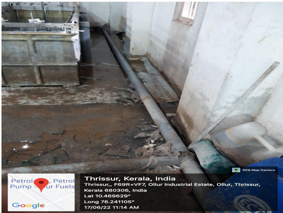
Figure 6 - Wastewater conveyed to the outside premises at Bright Precured Systems 2
