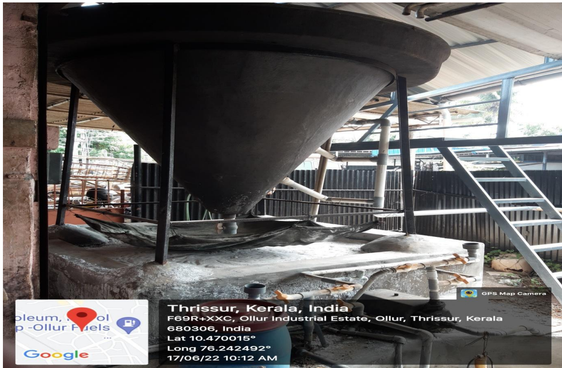
Figure 5 - Hopper bottom settling tank and sludge drying bed
