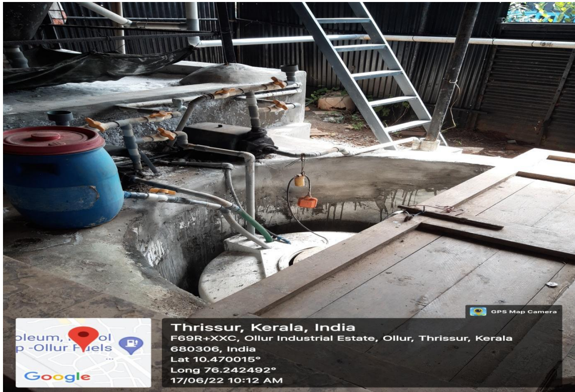
Figure 4 - Collection tank and chemical addition installations in ETP
