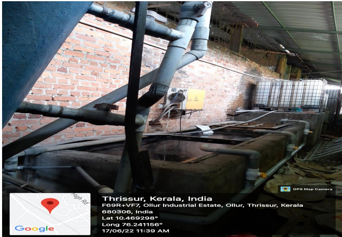
Figure 7 - Defunct effluent treatment plant at Bright Precured Systems 2
