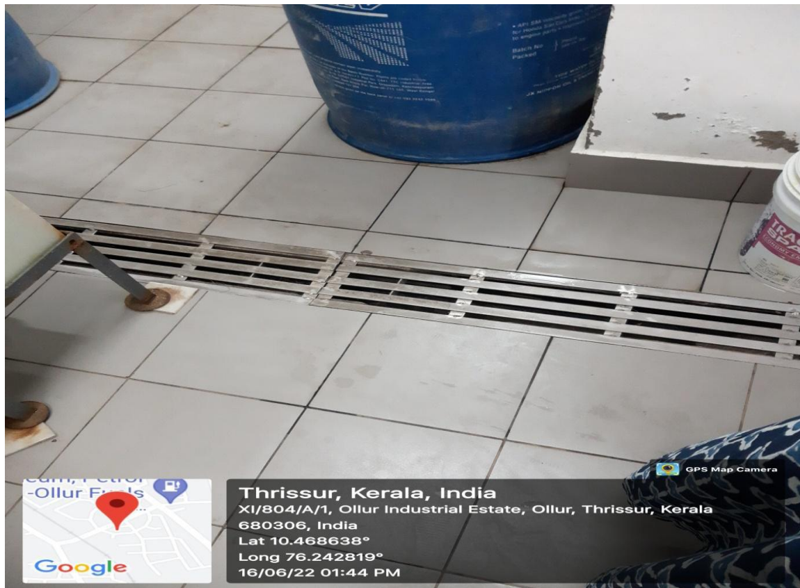
Figure 3 - Drains for conveying spillages to the effluent treatment plant
