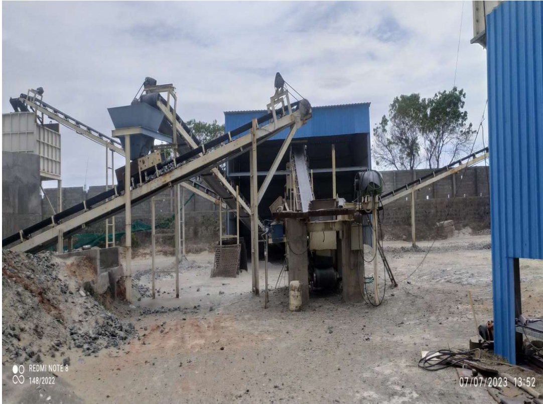
Conveyor connecting cone crusher and vibrating screen
