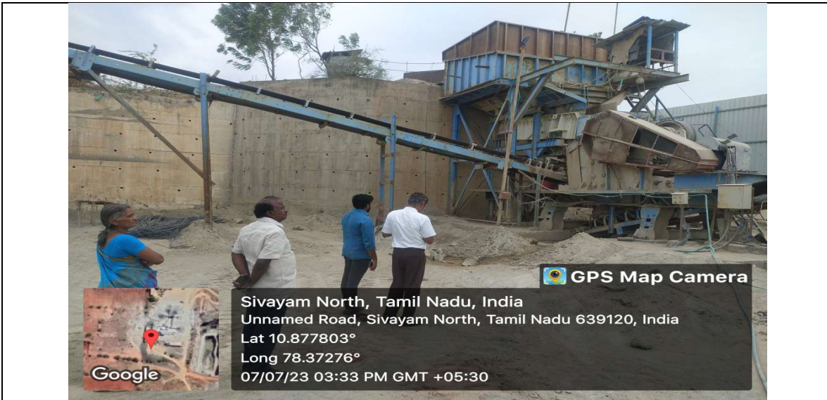
Water Sprinkler arrangement provided in Primary Crusher
