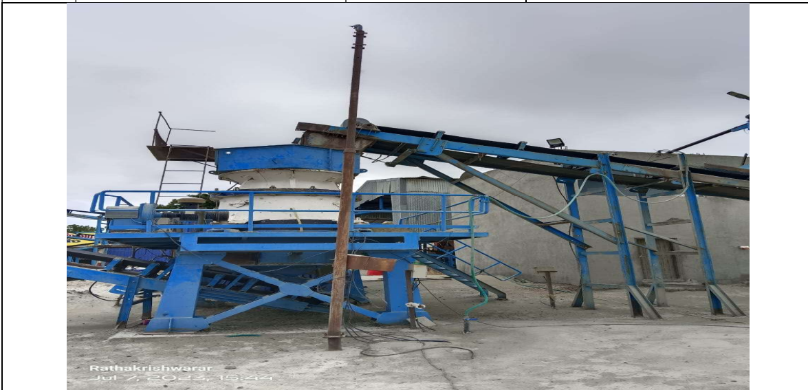
Cone crusher without GI Sheet Covered shed
