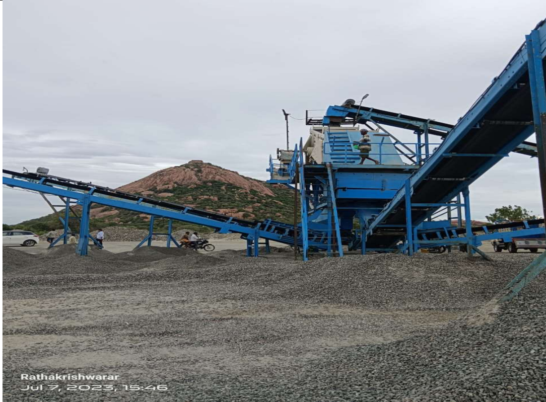
Vibrating screen and Conveyors without metal sheet cover
