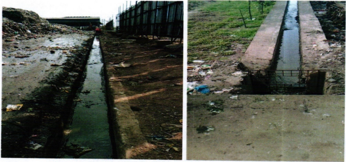
Separate drains (above photos) for collection of leachate generated from fresh waste processing areas such as Pre-sorting, compost plant, RDF storage etc
