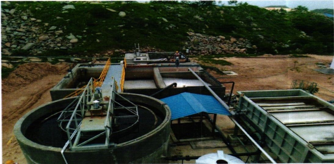
Pretreatment of Leachate (above)
