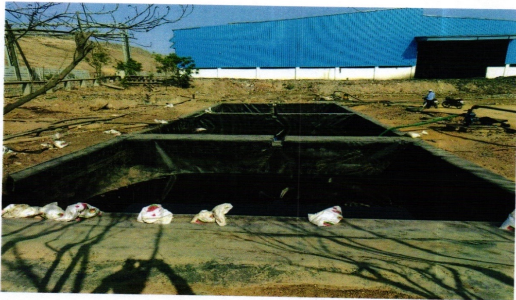
Leachate drains are connected to pumping ponds (above photograph) for pumping into larger capacity ponds before treatment
