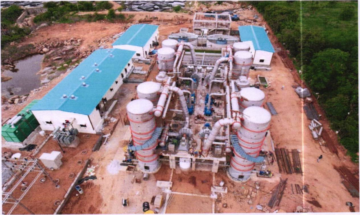
Legacy Leachate Treatment plant with MVRE Technology
