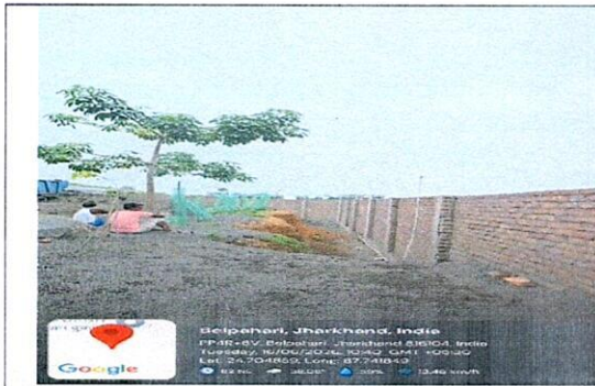
Fig. 11. Boundary wall and fixed type sprinklers
