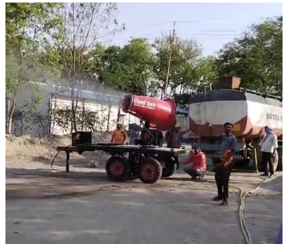
Fig 05- Fixed Type Water Sprinkler along Haul Road and Fog canon in Coal stock
