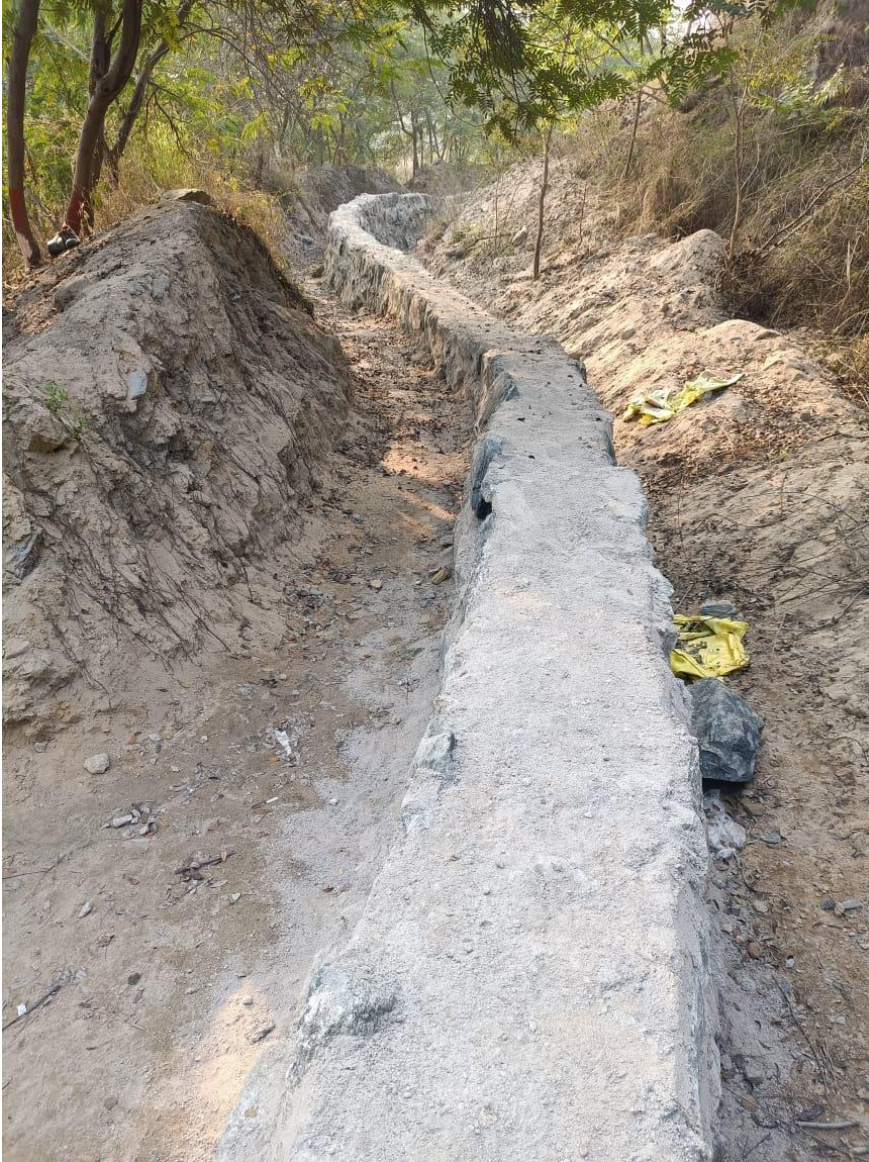
Fig 10 continuation- New toe wall constructed for 1200m along the tow of the dump
