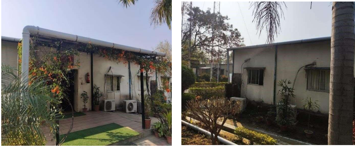
Fig 07 –Roof Top Direct Rainwater Harvesting Structure
