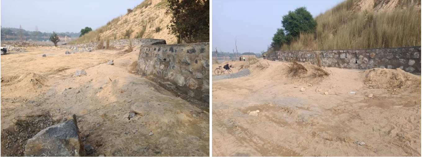
Fig 10.2: Continuation- New toe wall constructed for 1200m along the toe of the main dump
