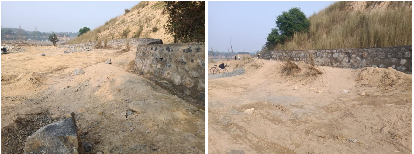
Fig 10.2: Continuation- New toe wall constructed for 1200m along the toe of the main dump
