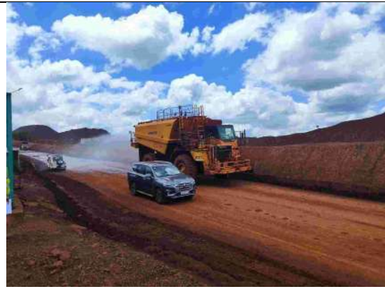
Photo 16: 50KL Water Sprinkler
