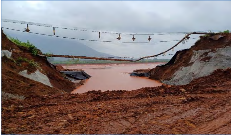
Figure-6 : Dyke Breach photograph
