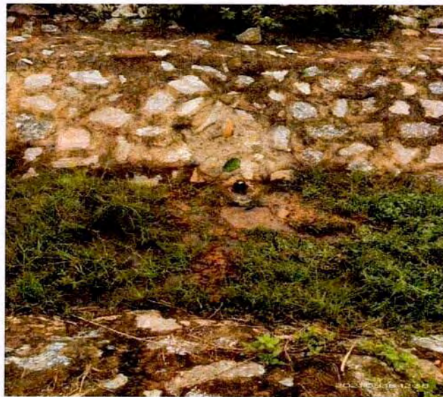
Fig. 5.4 Seepage location-2 between section A8-A9
