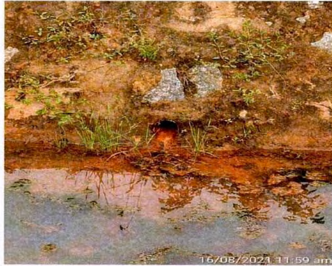
Fig. 5.3 Seepage point location 1 between section A8-A9
