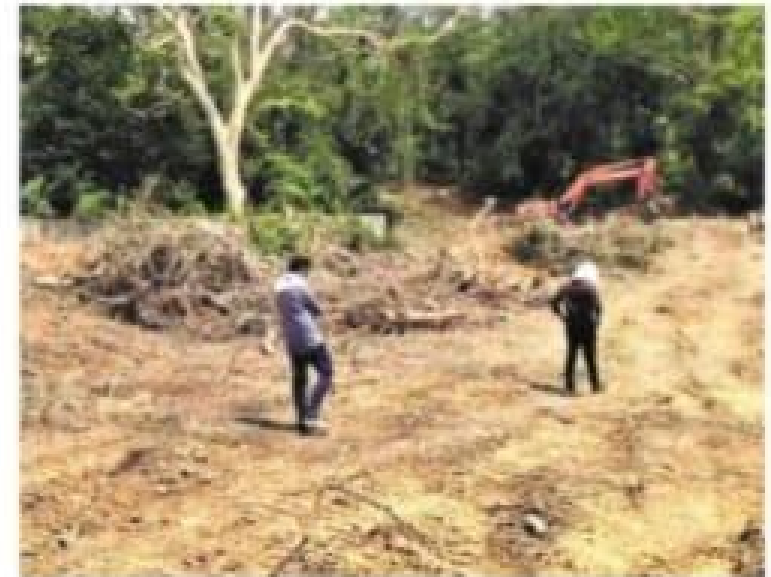
Felled trees being cleared from near Jhinjirband pond in Baripada town | EXPRESS
