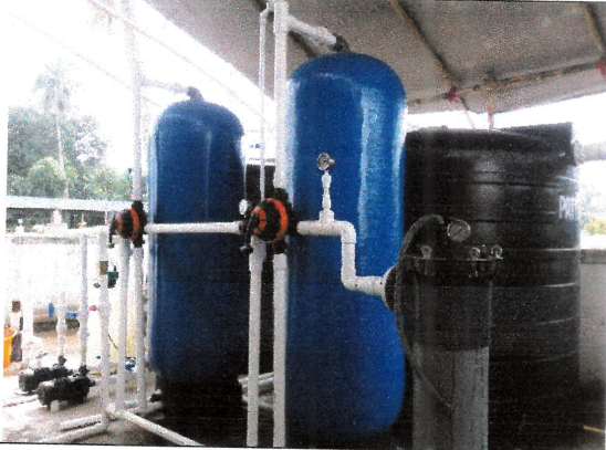
Pressure sand and activated carbon filter
