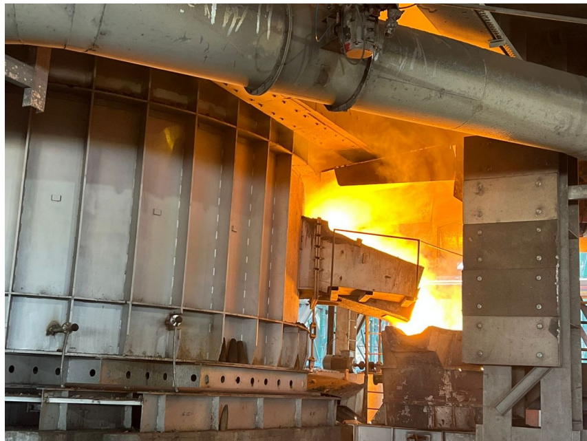
Photograph 6: Tapping point of metal is connected with APCD device
