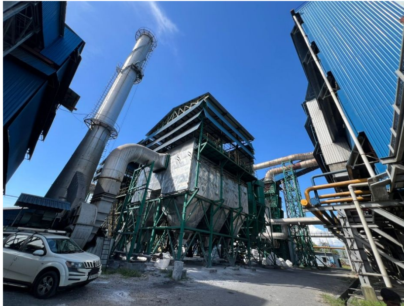
Photograph 1: APCD/GCP installed in M/s Aether Alloys LLP
