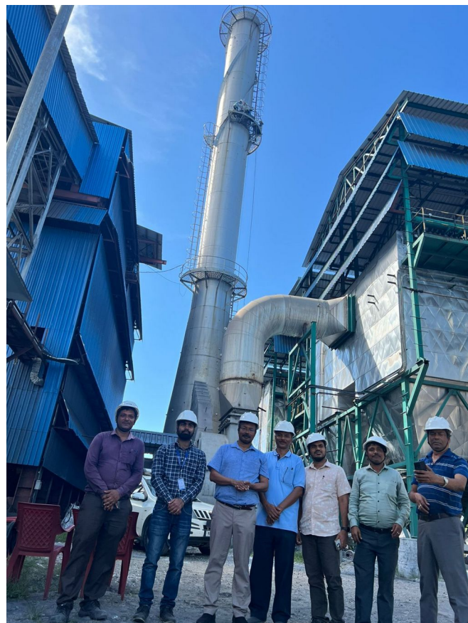
Photograph 2: Chimney of 40m high connected with APCD/GCP
