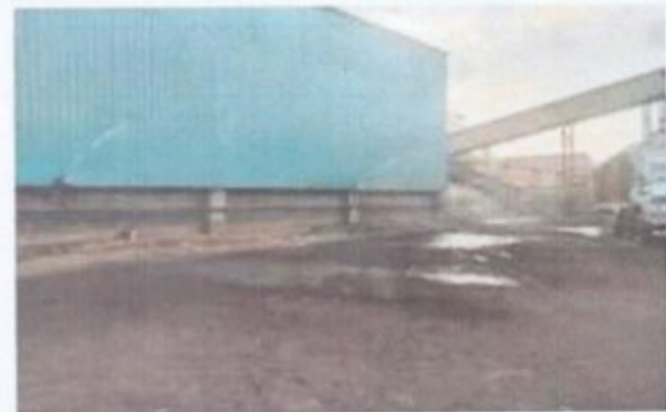
Fixed rotary type water sprinklers
