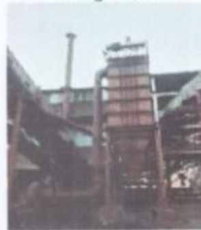
Iron Crusher Bag filter
