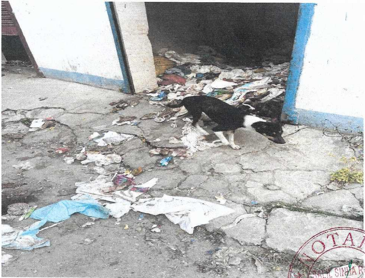
Photograph taken on 02/12/2025 showing the biomedical wastes inside the designated storage rooms of Alipurduar District Hospital
