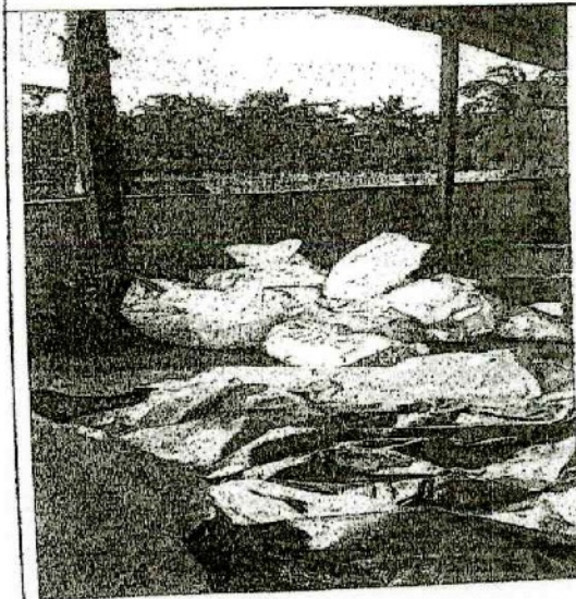
Pic-3(New Hazardous Waste Storage Shed, not properly covered)
