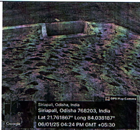
Holding tank of the garland drain around the Tailing Pond No. 2
