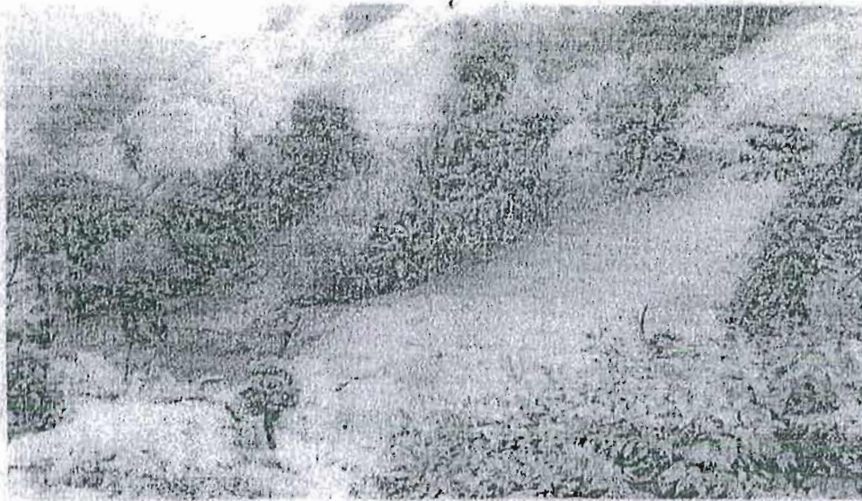
Picture-1. Indiscriminate dumping of muck/debris in the project site by Shivam Trans Construction Private Limited. The muck/debris are seen rolling down the hill slopes in total violation of the guidelines of the Forest Clearance and making a mockery of the Designated Dumping site guidelines.
