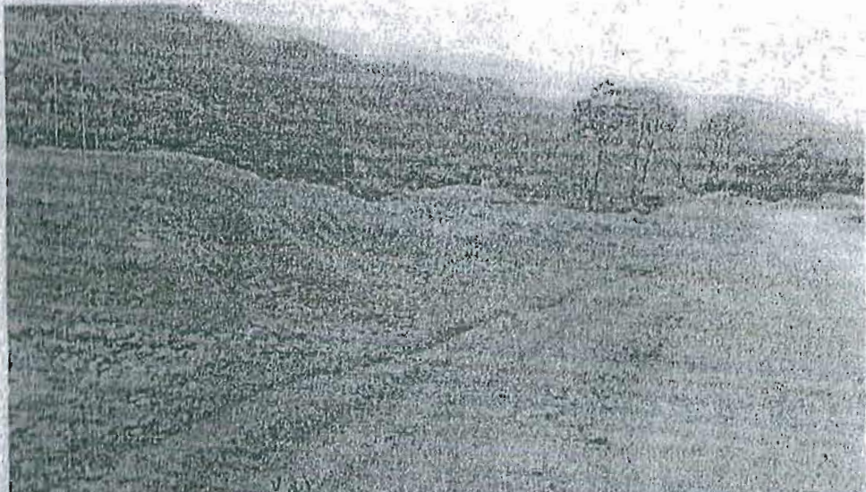
Picture:4: The muck being along the road side in flagrant violation of Muck Disposal Plan issued to Shivam Trans Construction Private Limited. These muck roll down the hilly slope and also the dust emitted from these muck make the life of commuters a hell.
