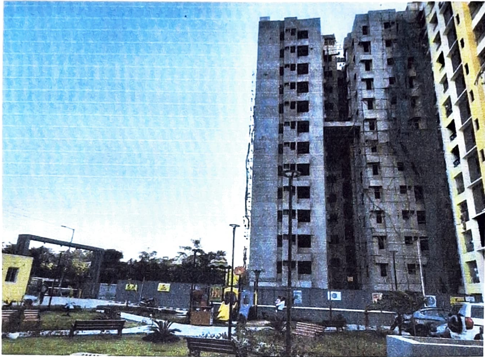
Pic.6: Construction work going on at the time of field visit in TARANG portion of the project
