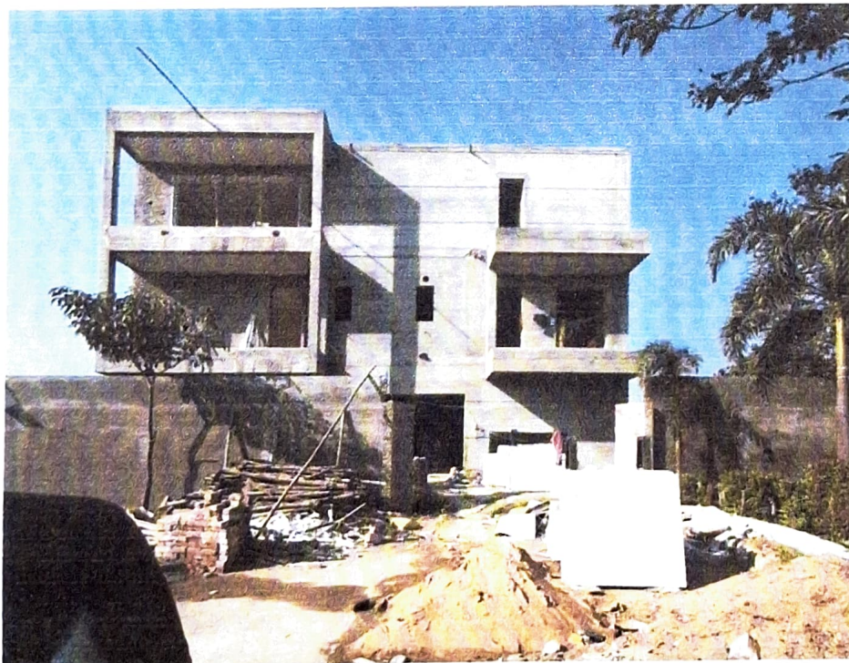
Pic.5: Construction work going on at the time of field visit in individual plots in Phase- IC (TOWNHOUSE)
