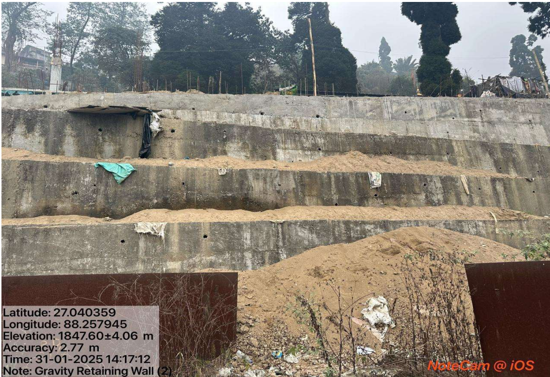
R.C.C COUNTERFORT RETAINING WALL OF 6.50m HEIGHT CONSIDERING WITH SUPERIMPOSED TRAFFIC LOAD ALONG THE APPROACH ROAD
