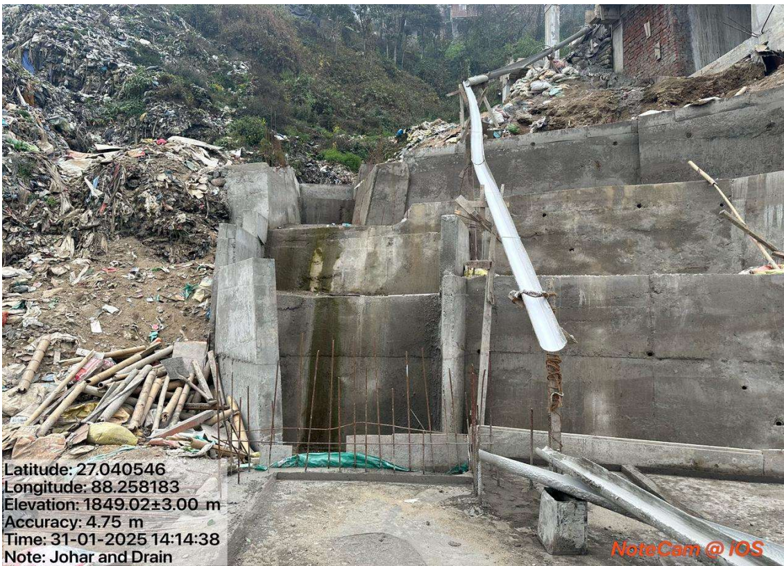
JHORA (DROP GUIDE) AND STORM WATER
