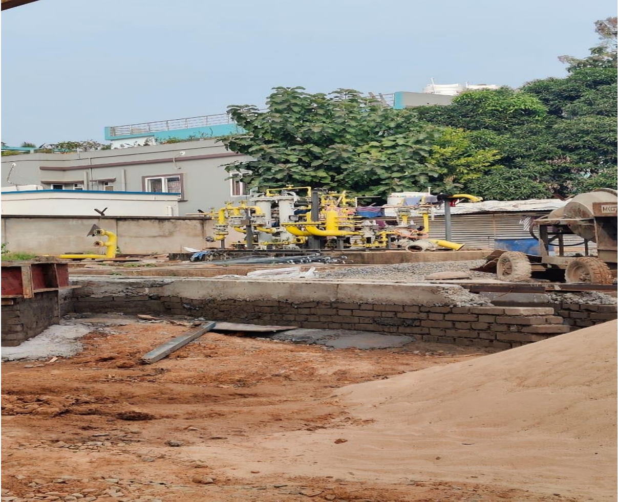
PHOTOGRAPH DATED 26/11/2024 SHOWING LARGE SCALE CONSTRUCTION OF CNG STATION IN CLOSE PROXIMITY OF RESIDENTIAL HOUSE.
