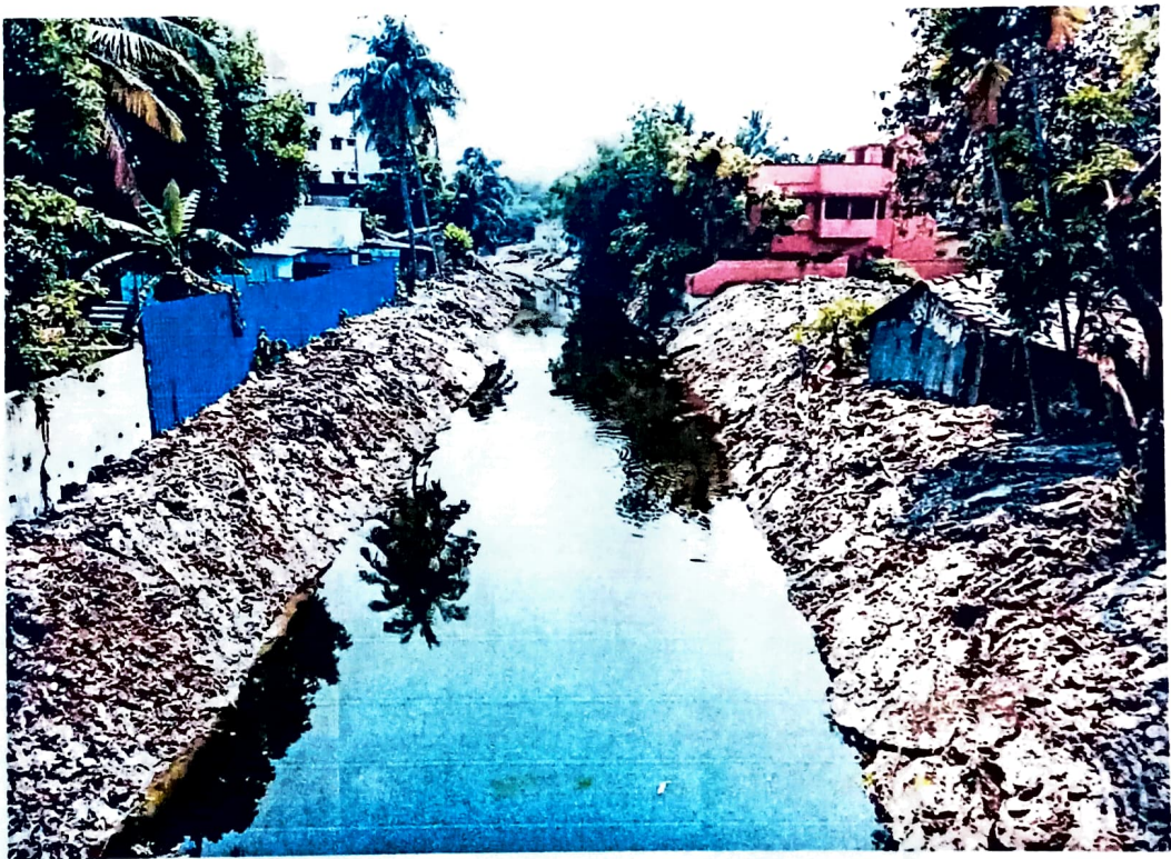
After Cutting at Down Stream of Howrah – Kharagpur S.E.Rail Line , Masila Bridge.
