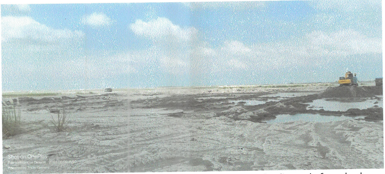
Figure 4 Photos of the ash pond showing different activities for disposal of pond ash.
