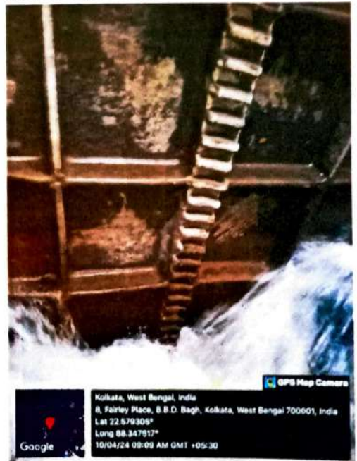
Jackson Ghat Penstock Gate
