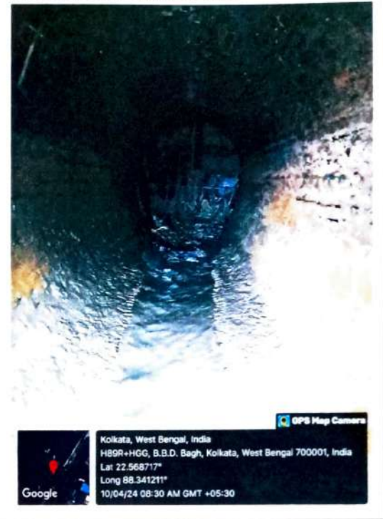
Chandpal Ghat Penstock Gate
