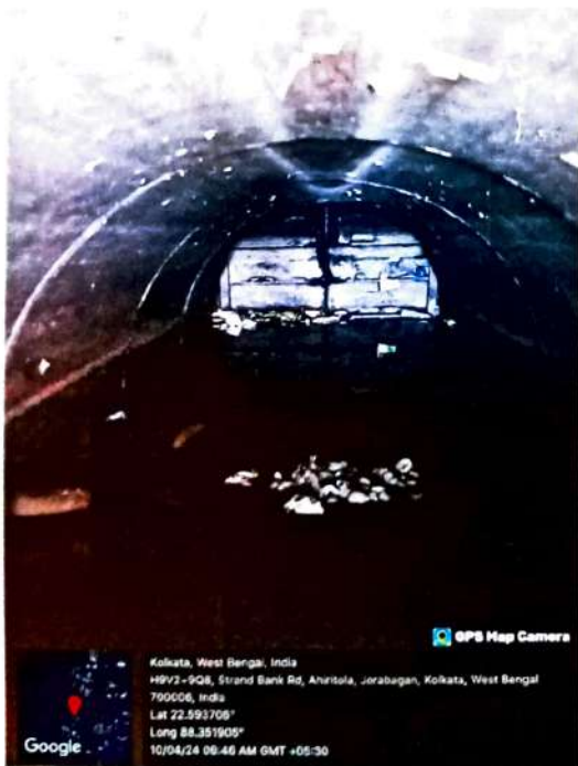
Nimtola Ghat Penstock Gate
