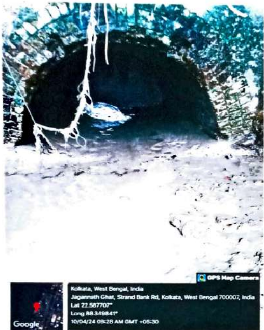
Jagannath Ghat Penstock Gate
