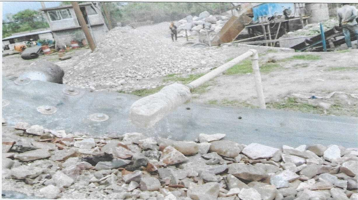
Picture: Provision for water sprinkling at M/s Shri Balaji Minerals (Stone Crusher) at Moruk area, Mebo , East Siang District, Arunachal Pradesh.
