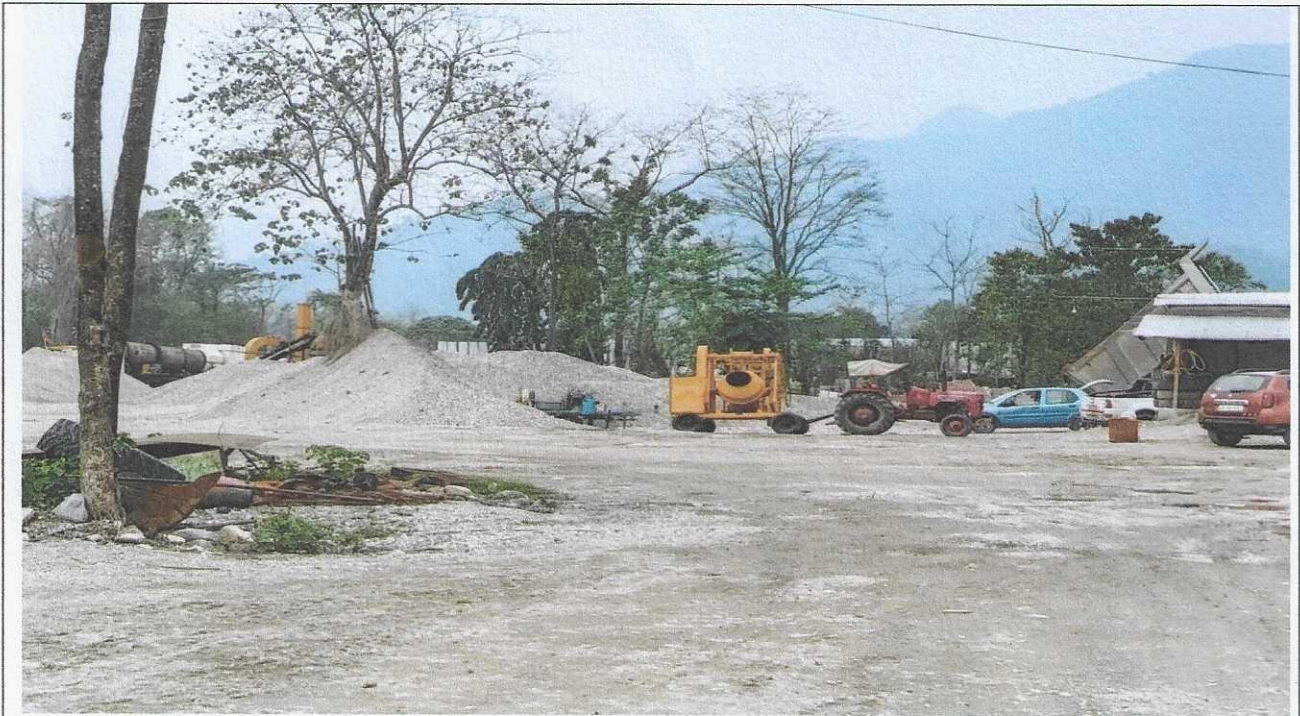
Picture: Camp of M/s Shri Balaji Minerals (Stone crusher) at Moruk area under Mebo Circle, East Siang district, Arunachal Pradesh.
