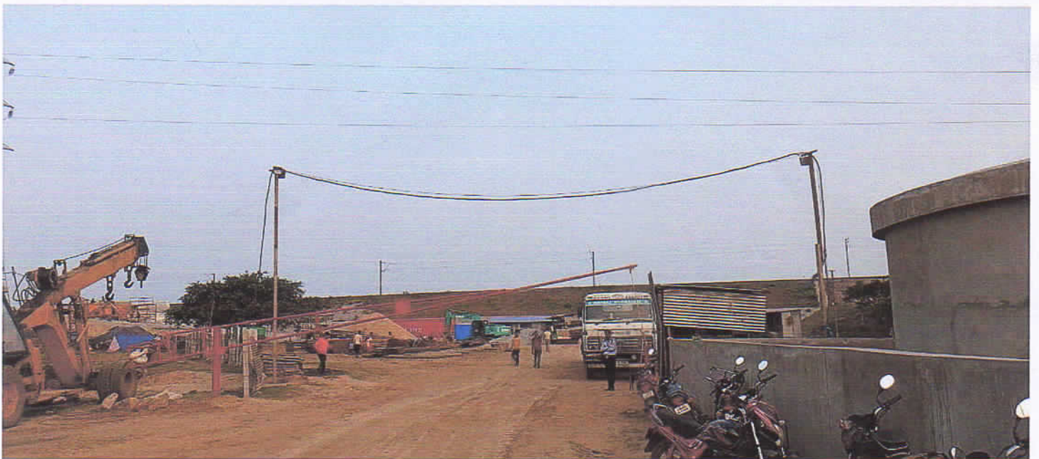
Photo Copy :Construction site camps and Batching Plants and different minor minerals dumped by M/S Rajbir Construction pvt.Ltd .Jharkhanda.Plot No 705/861 of Khata-No-330 of Mouza Badapal, Kism Nadi having area 18.74 Acres Under Marshaghai Tahasil of Kendrapara Dist.
