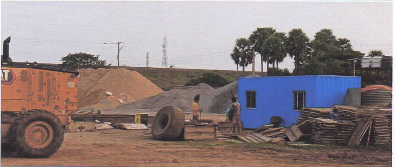
:Photo Copy ;Construction site camps and Batching Plants and different minor minerals dumped by M/S Rajbir Construction pvt.Ltd .Jharkhanda.Plot No 333 of Khata-No-333 of Mouza Badapal, Kisam Nayanajori having area 21.06 Acres Wornership which bilongs to Nirman (PWD) &Paribahan (Transport) Dept Under Marshaghai Tahasil of Kendrapara Dist.
