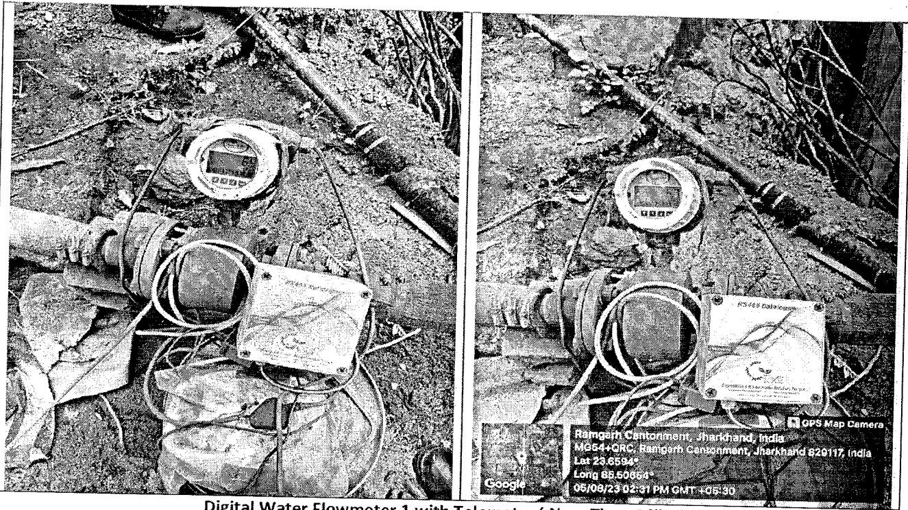
Digital Water Flowmeter 1 with Telemetry ( Near Time Office)
