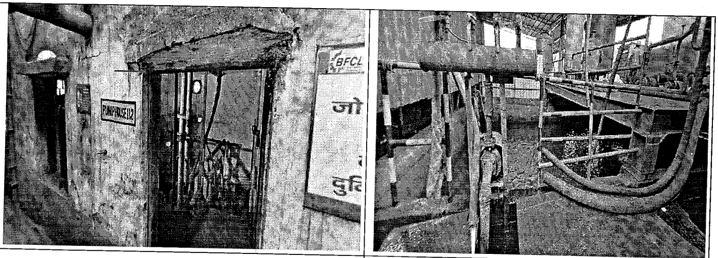
Pump House(1st & 2nd)
