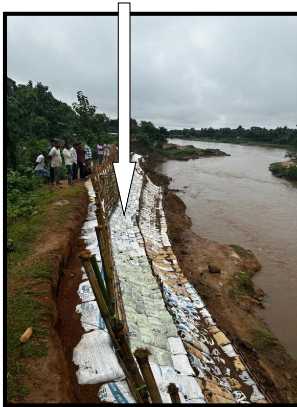
PLATE – II (PIC SHOWING PARASIDING AND SAND FILLED BAG WITH BAMBOO SUPPORT ON BOTH SIDE OF RONGAI RIVER)
