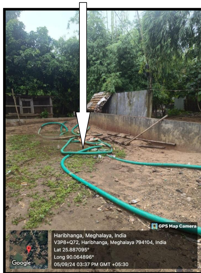
PLATE – III (PIC SHOWING RIVER SAND HEAP, STORAGE SPACE & WATER PUMP WITH PVC PIPE)
