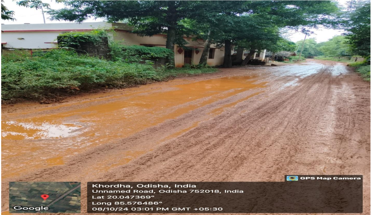
PHOTOGRAPH DATED 08/10/2024 SHOWING CONDITION OF THE ROAD
