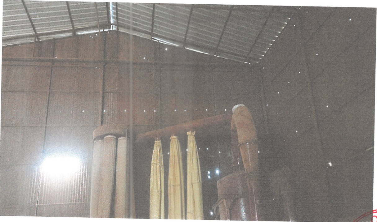
Holes in the shed observed which serve as dust leakage points
