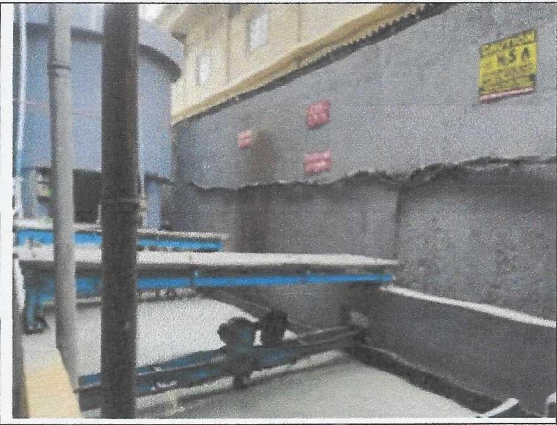
Fig. 11: Effluent Collection Tank at Tannery
