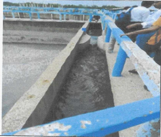
Fig. 6: Parshall Flume after Sulphide Tank
