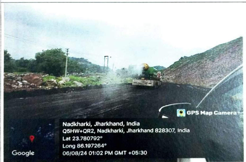
Pic 5 & 6: Water sprinkling on major roads using water tanker and mist cannon
