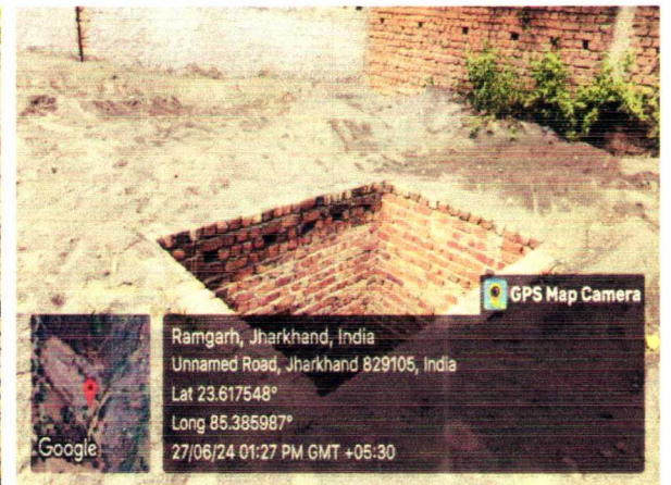
Photo 44: Photo of other siltation pond inside the unit premises.
