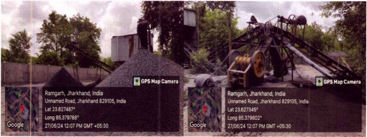
Photos 7 & 8: Photo of water spraying arrangements over conveyor belt and transfer points.
