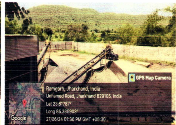
Photo 48: Photo of water sprinkling arrangement over conveyor belt transfer point.
