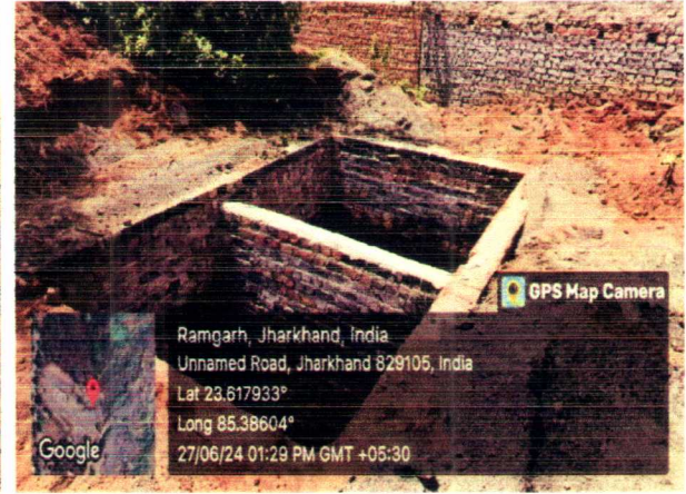
Photo 42: Photo of siltation ponds in the unit premises
