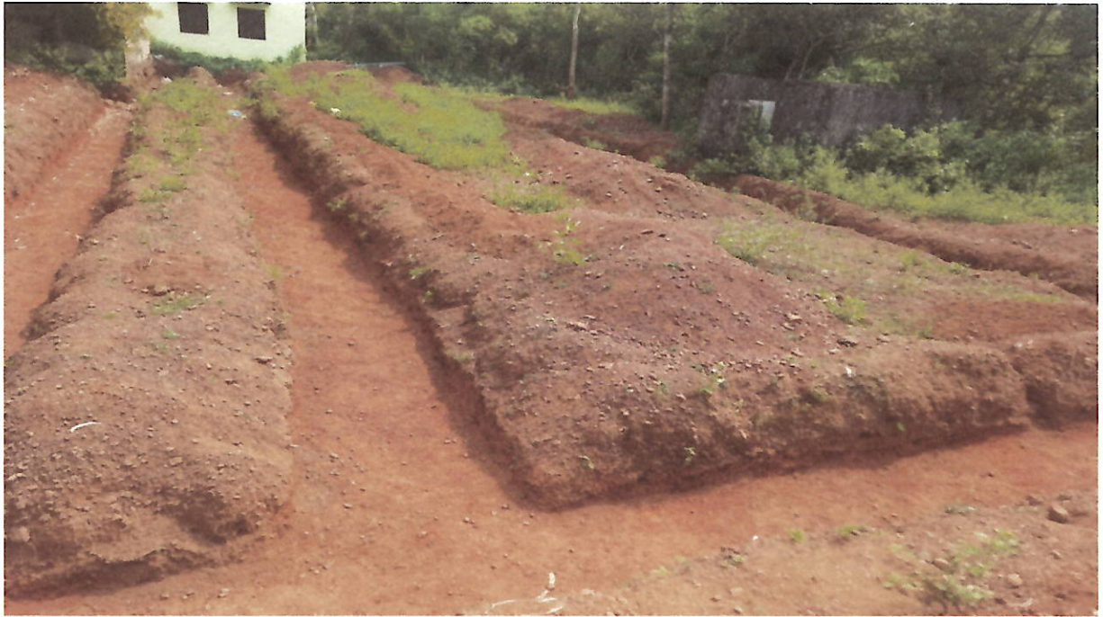
Const. Of conference Hall at Chintamani Vidya Niketana, Narangarh (Work on progress )
