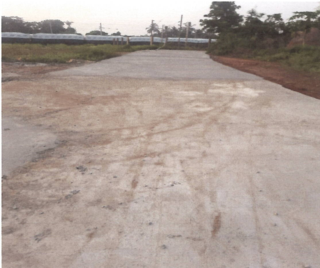
Repairing of CC road from Bhogapur mangala temple to Railway staff quarter (Completed)
