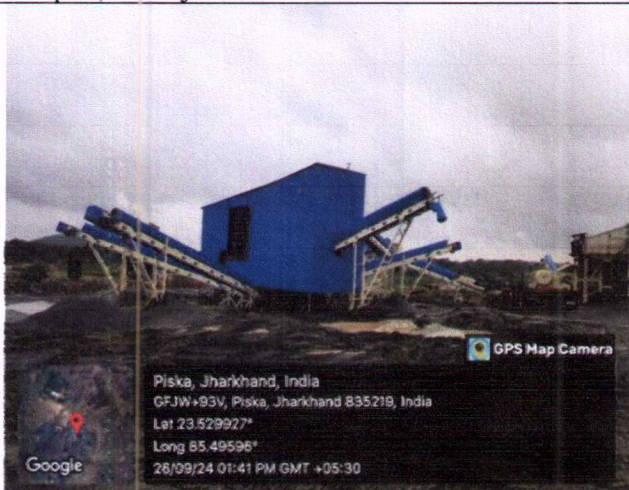
Photo 7: Covered conveyor belt and screen of M/s Bansidhar Construction Private Limited Stone Crusher unit at Piska, Ormanjhi
