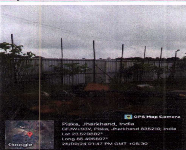
Photo 9: Metal sheet boundary wall constructed at M/s Bansidhar Construction Private Limited Stone Crusher unit in Piska, Ormanjhi
