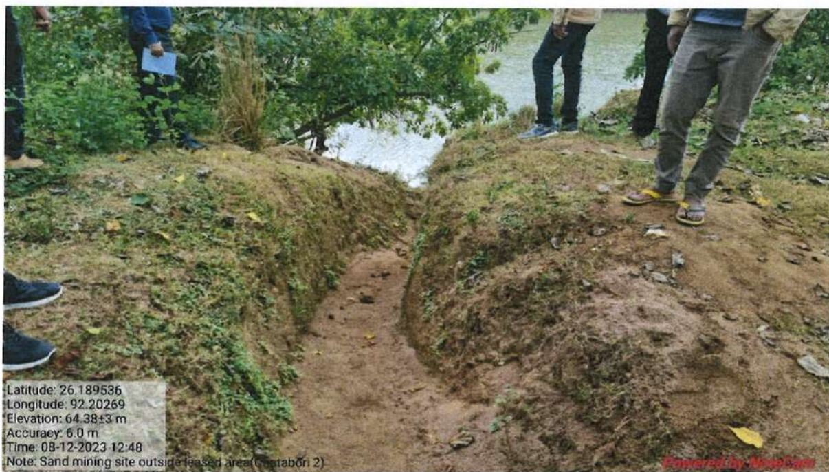
Fig.8a. A ramp has been constructed on the riverbank to facilitate the transportation of sand from the riverbed to the dumping site.
