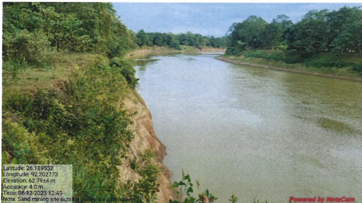
Fig.6. Erosion prone nature of the bank is shown by the steep bank at several places.
