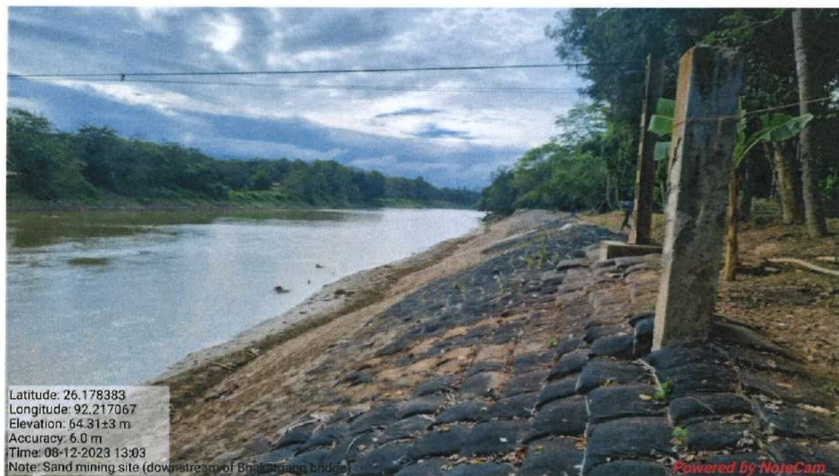
Fig.4. Bank protection measures (geobag) on the right bank of the river immediate downstream of the Bhakatgaon bridge and upstream of the Naokhola permit area.
