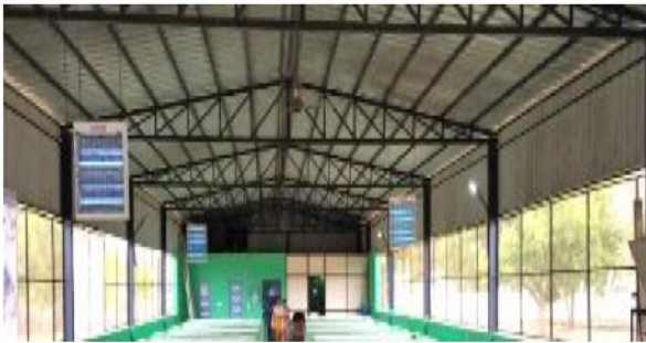
Figure 12: Fly traps installed at MCC
